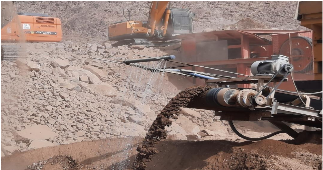
Figure 4. Crusher with water sprinkler system.
